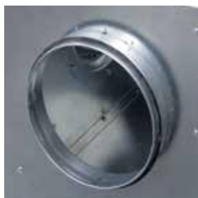
Rubber seals in the exhaust valves.
